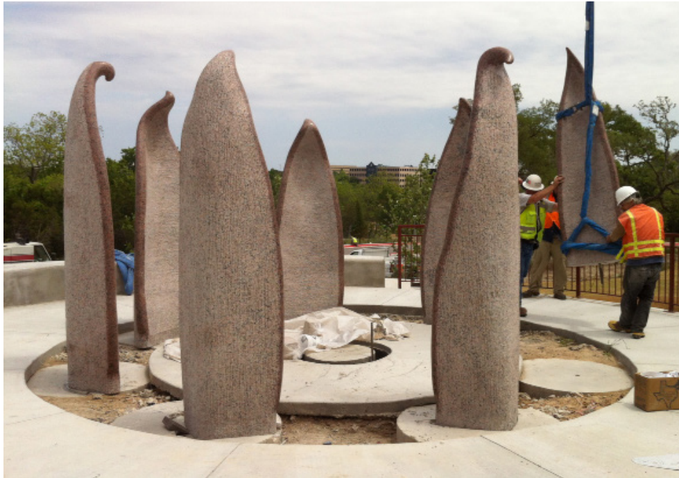
AIPP commissioned artist Philippe Klinefelter installing his carved granite pieces as part of Lotus , located at the Asian American Resource Center, with the help of a crane. The artist and all artist subcontractors must be insured in accordance with City of Austin policy.
